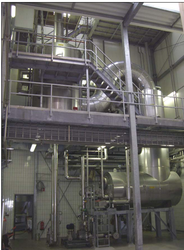
Figure 7. C & D, Packed column deacidification plant
